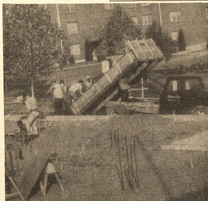
WORK PROGRESSES ON SCHEDULE on the half-million dollar men's dormitory which will be completed by next September.
