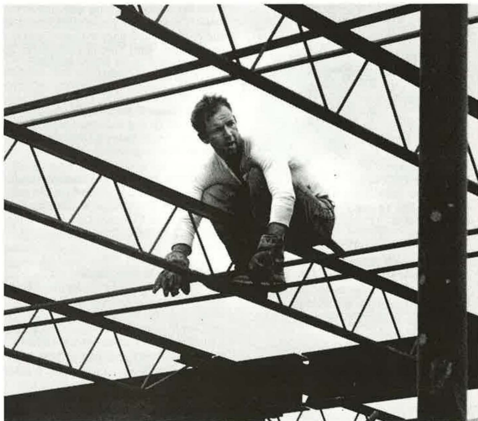
A construction worker has a lofty perch as he secures the steel undergirding for the roof of the new library facility which will be completed in July.
