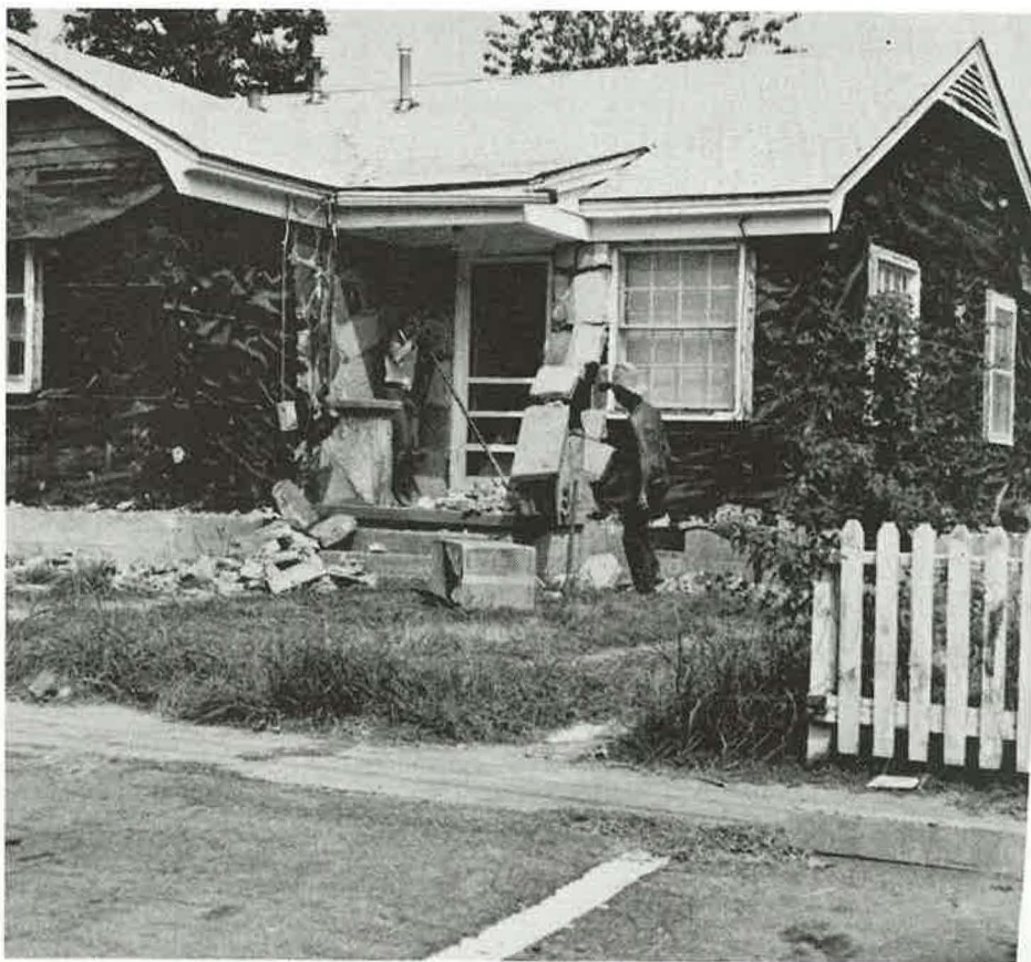
The rock houses on Blakeney Street just south of Rhodes Field House are razed to make room for construction of a new men's residence hall, scheduled for completion by the fall of 1989.
