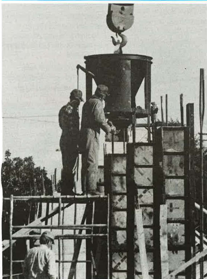
Construction began in September for a new men's residence hall, scheduled for completion in August.
