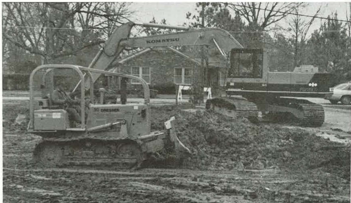
Foundation preparations began in mid-March for the addition to the Heritage cafeteria, which will give it a seating capacity of 1,100 when it opens for use this fall.
