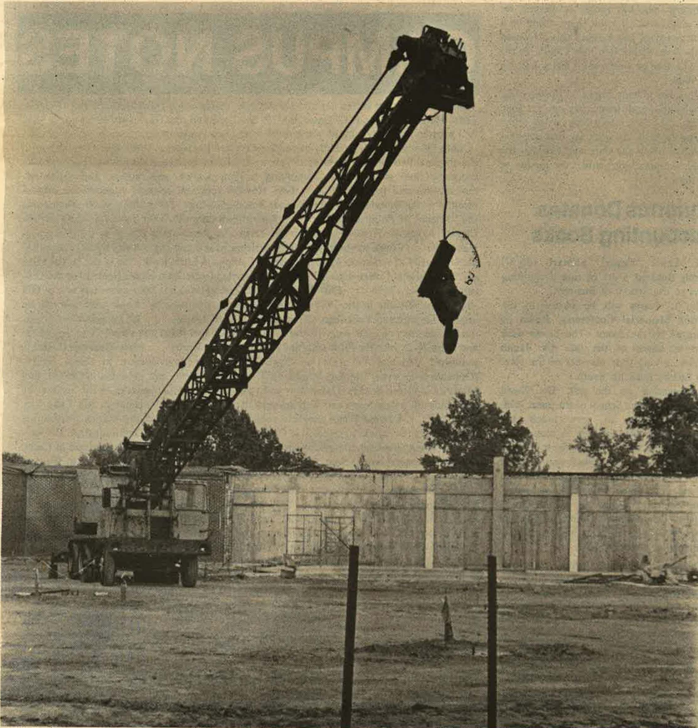
Construction work has begun on the $1.1 million, 14,600 square feet Science Building addition. (Photo by Bruce Cook)
