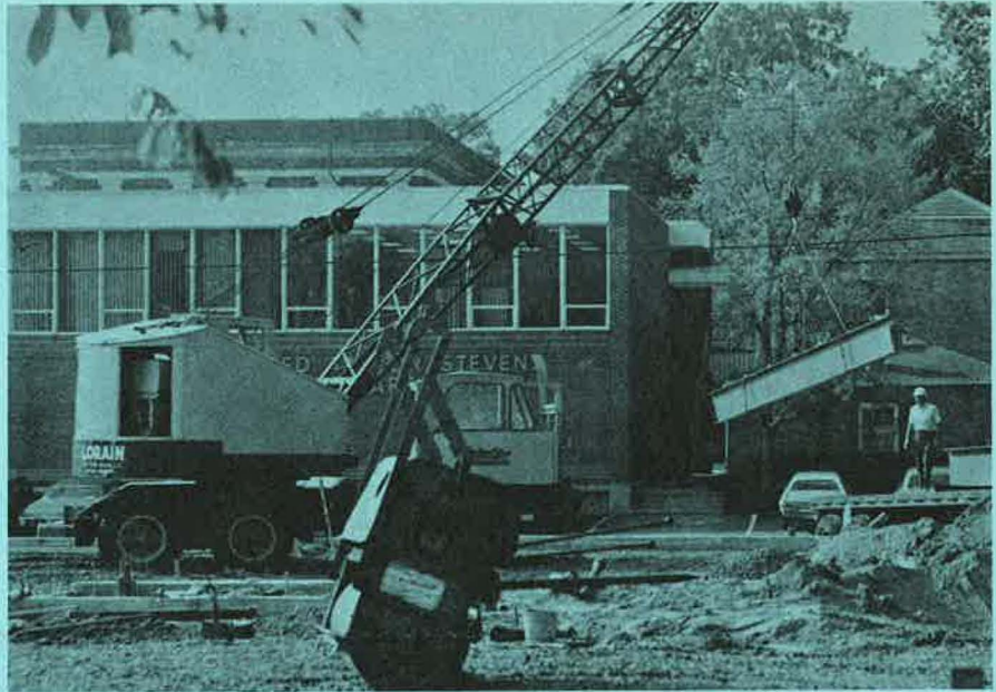
Workmen unload steel girders which will be used in the construction of the new $850,000 student center. Construction is expected to be completed by the fall semester of 1973.
