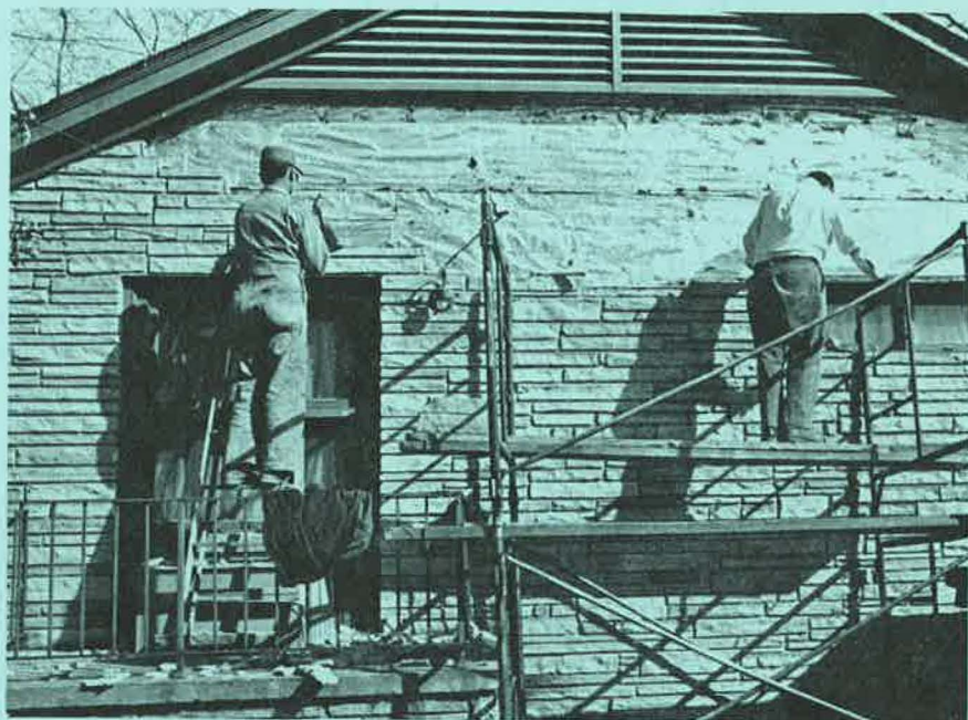
INITIAL STEP — Before construction on the student center could begin, three houses were moved. Above, workmen remove the rock from the exterior of the home of Dr. Jack Wood Sears. The Sears' home was moved to a lot on East Market Street.
