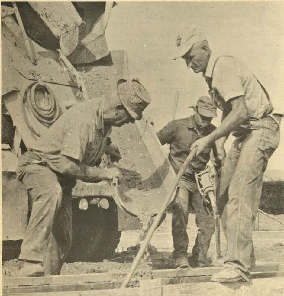
POURING THE FOUNDATION — Workmen pour the cement into the wooden forms of the new men's dormitory. The $975,000 structure is scheduled for completion in September, 1971.
