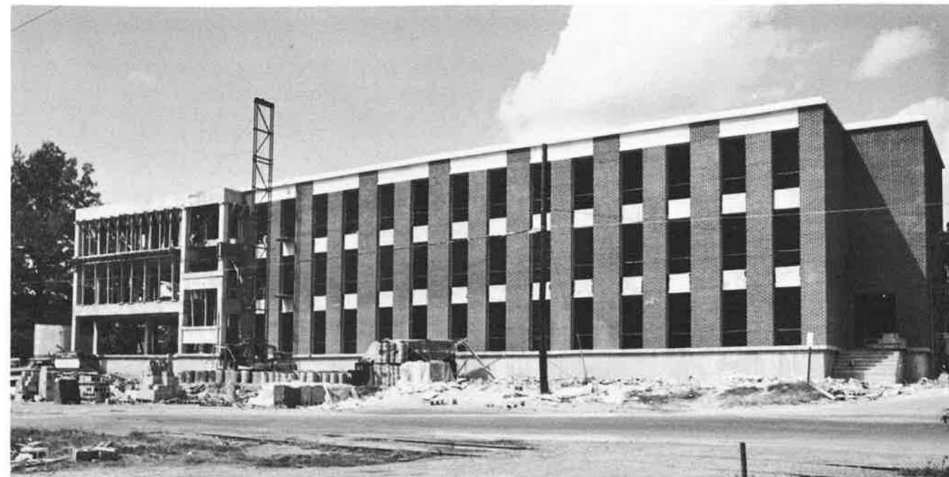
SHAPING UP—The last of the concrete superstructure of the new women's dorm was completed in July. What can be seen through obstructions gives an idea of the massiveness of the new home for 234 women scheduled for occupancy in January, 1968.
