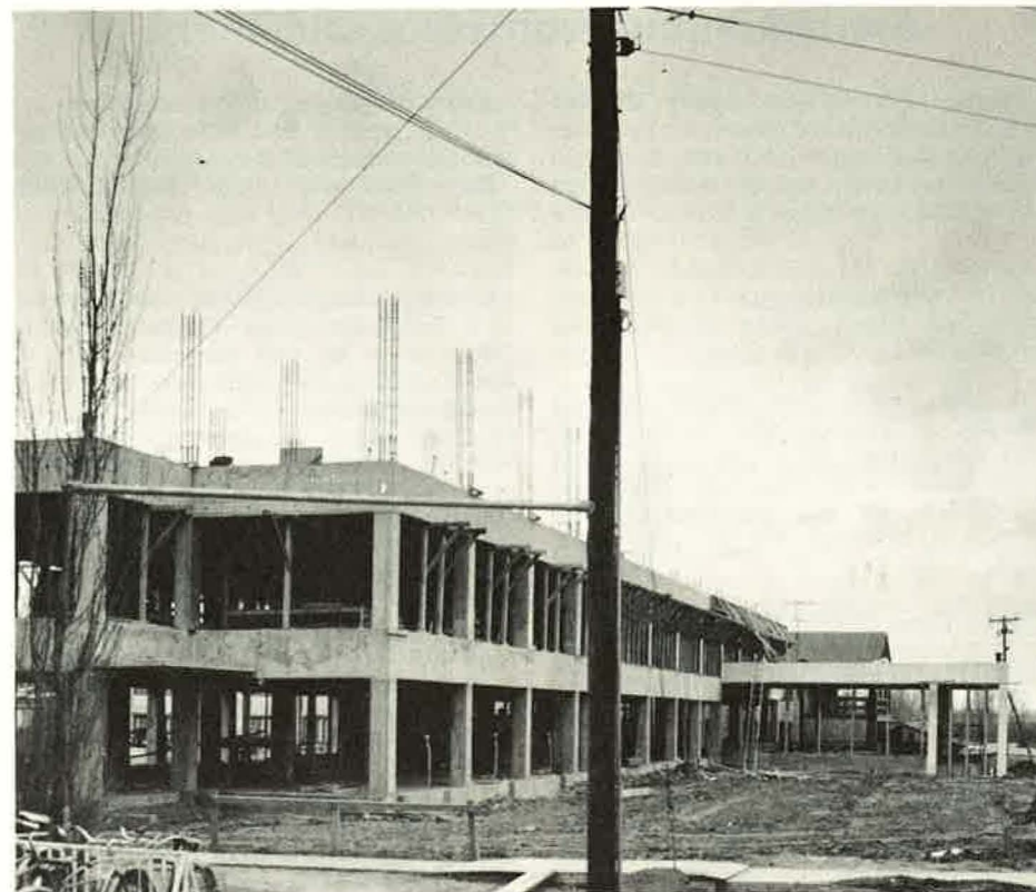
Construction continues on the new boys' dormitory despite subfreezing temperatures of a January in Arkansas. The dormitory is scheduled to be completed during the summer and will be ready for occupancy in the fall — marking the first all air-conditioned dormitory on campus.
