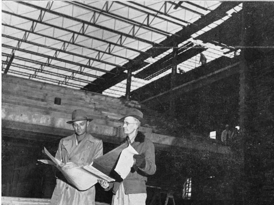
Top: Workmen are welding steel decking for the roof of the auditorium-administration building. Bottom: Garner (left) and Wallace check the blueprint on a construction problem.
