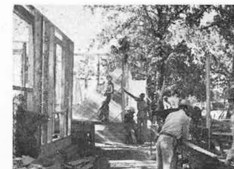
Student helps nail on timbers in housing project, as Mr. Earl Smith operates power saw.
