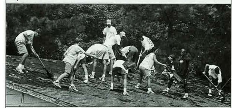
During a Student Impact service project the first week of school, students help dismantle a building the city of Searcy needed removed from Spring Park.
