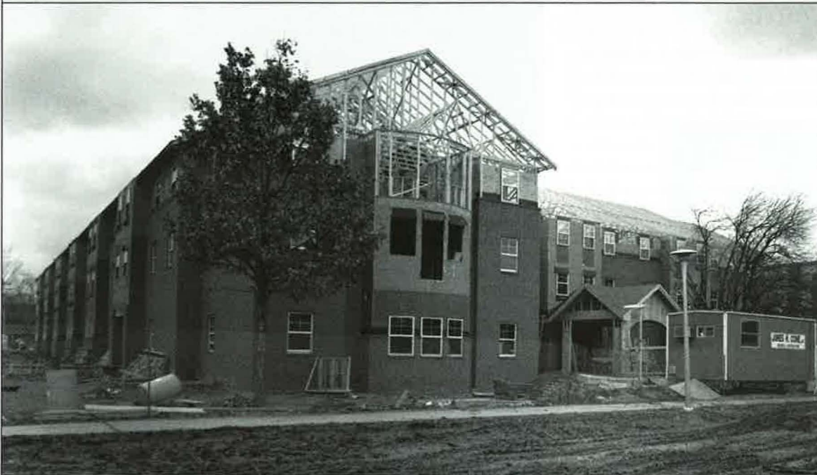
Construction on the new women's apartment-style residence hall at the corner of Center and Remington streets is proceeding on schedule and will be ready for the start of the fall semester. The facility will house 196 women and features four-bedroom suites.
