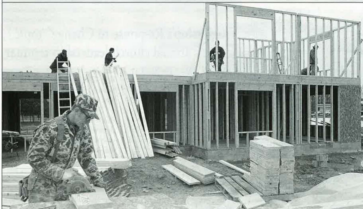
Construction has begun on the new married-student apartments located at the corner of Benton and Park streets. The complex is scheduled for completion in August by the beginning of the fall semester.
