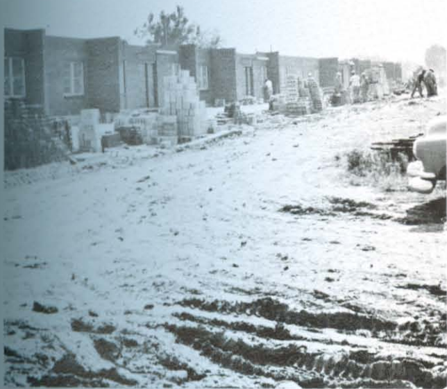
WITH some in skeleton form and some ready for occupancy, the modern buildings in Vet Village will soon house married students.
