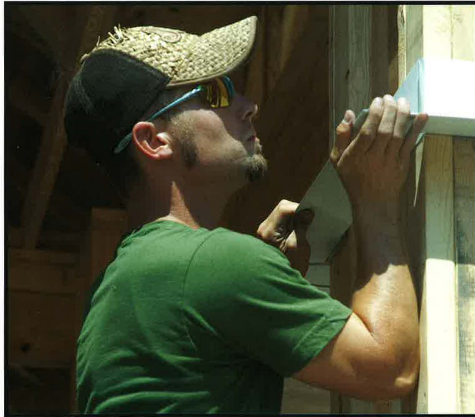
Damon Pearrow works on constructing the support columns outside the main entrance to Sears Hall.
