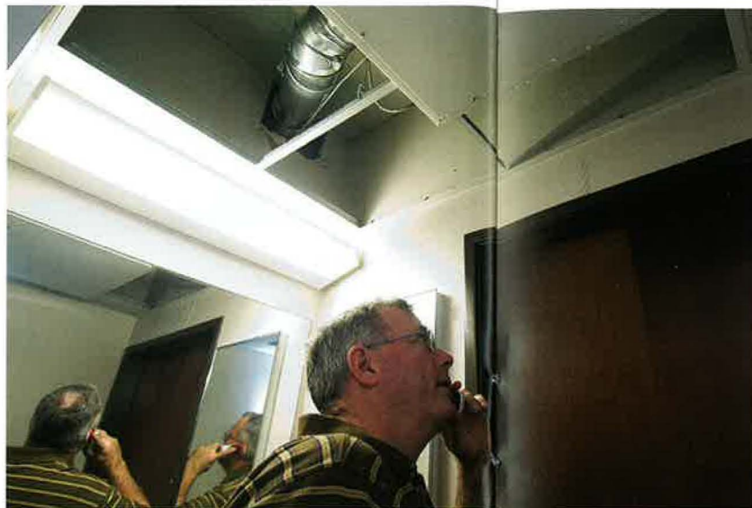
An early morning air conditioning problem in Allen Hall finds Dana McMillion, director of maintenance, on the job. PHOTO BY JEFF MONTGOMERY
